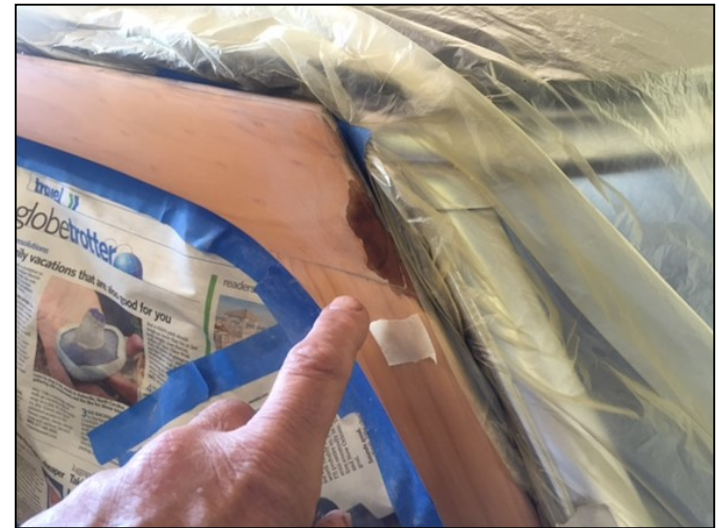
Wood with unrepaired water stain
