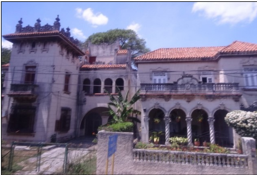
This is a very nice home in Cuba that has fallen into disrepair. It was a private home under Batista. We were told that the government was going to repair it, but as usual there are no funds available. We were also told on the tour that when completed, it would go to some government official.
